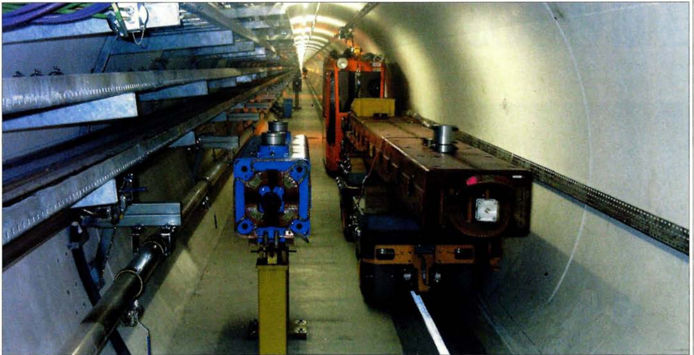
Transport convoy carrying a main dipole in the straight part of TI 8, during the initial phase of the installation. The set of engines automatically followed the white guidance line and attained a typical driving speed of around 3.5 km/h.
