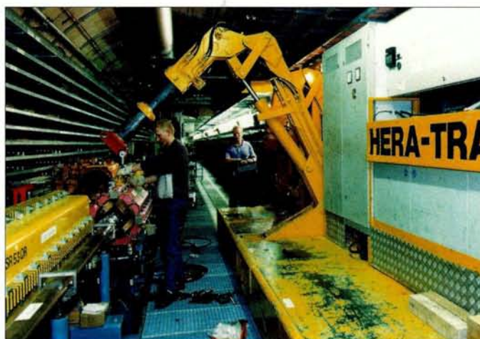
Nearly 80 new magnets – each weighing up to 7 t – were installed in HERA's proton and electron accelerators during the luminosity upgrade from September 2000 to July 2001.
